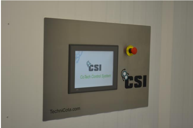
Example of control panel
